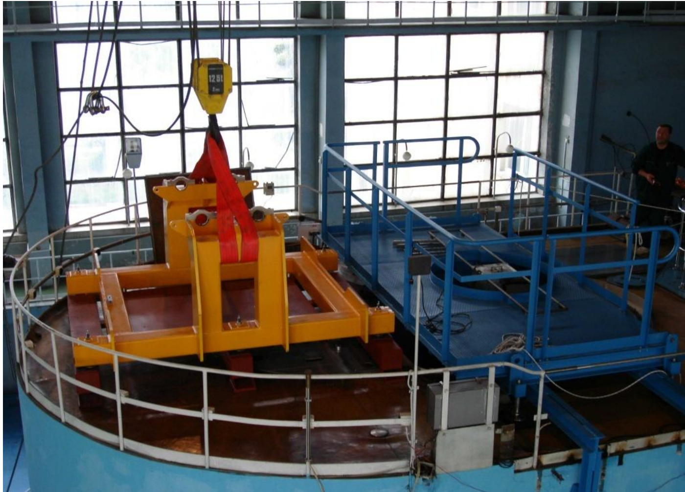
Bulgaria: cask manipulation platform on the reactor top
