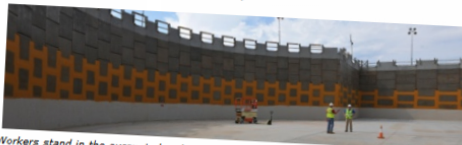
Workers stand in the excavated and waterproofed space for Vogtle 3's reactor building (Image: Southern)
