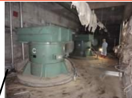
EDG air blower
