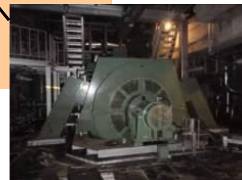
Emergency Diesel Generator (EDG)
