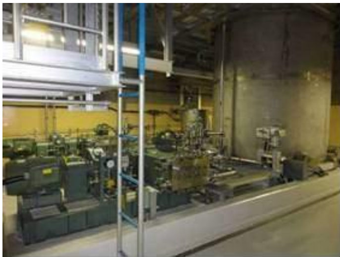
Pump and tank of Stand-by Liquid Control system
