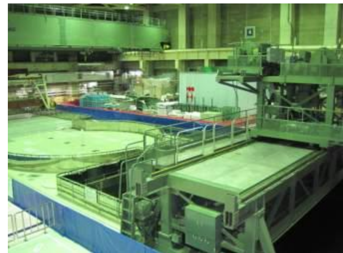
Reactor refueling floor
