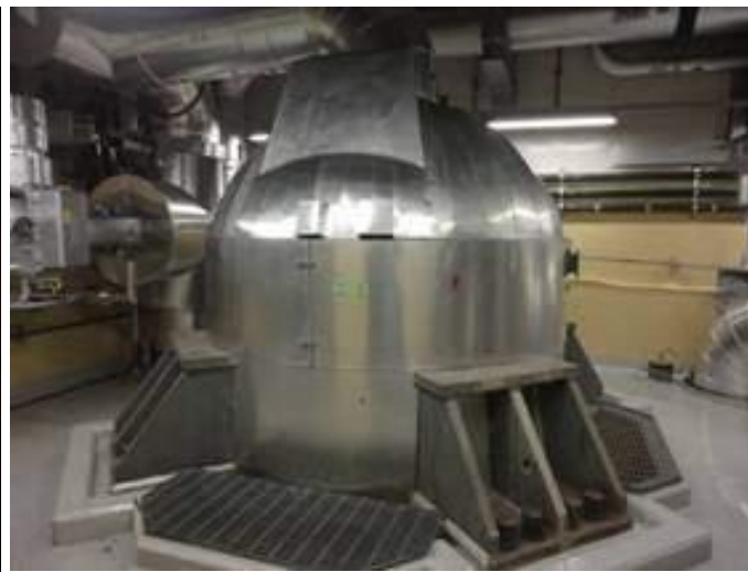
RHR heat exchanger
