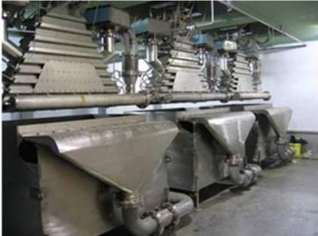
ELV-12 three-head beam extraction system at dyeing factory in South Korea. The productivity of the system is 10,000 m 3 /hour
