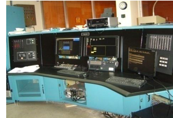
Digital control console
