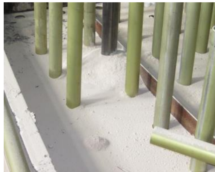
Void-free filling of reactor space by barrier materials. Result of the mock-up testing.
