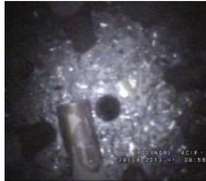
Performance of technological channels through metal constrictions of the lower biologic shield
