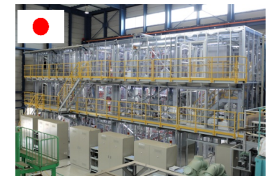
Hydrogen production test facility
